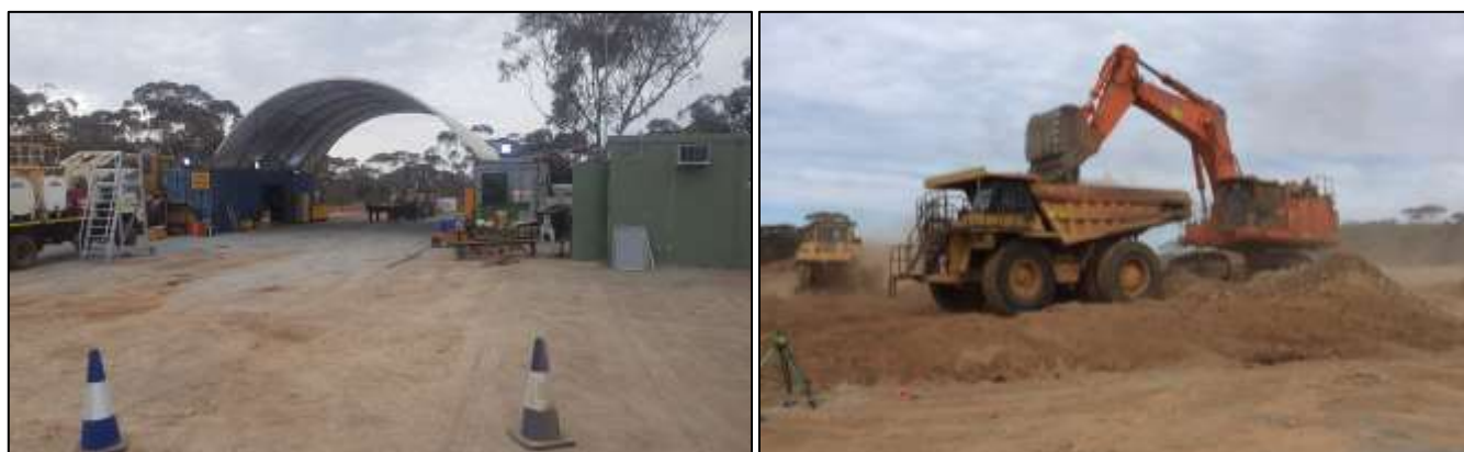
Photo 2A: Hampton workshop set up; Photo 2B: First waste loading at Flinders Main pit
