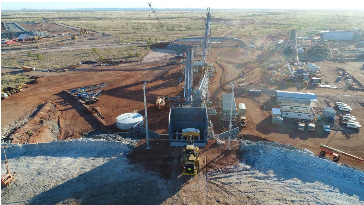
Ore Load Commissioning at Crushing Facilities (Figure 1)
